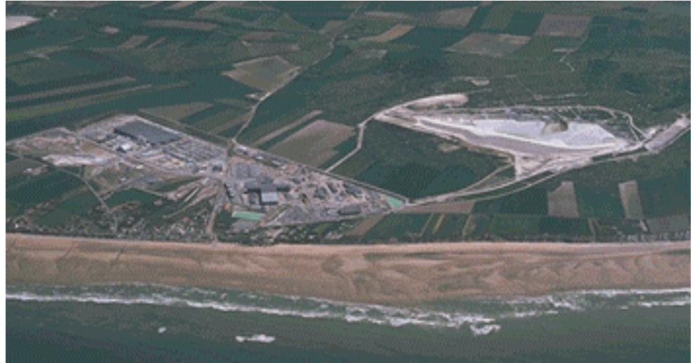
Sangatte Shaft during construction - From left to right: Precast plant, segments storage yard, Shaft under its temporary cover, maintenance and other temporary workshops, water treatment plant, and Fond Pignon Dam
